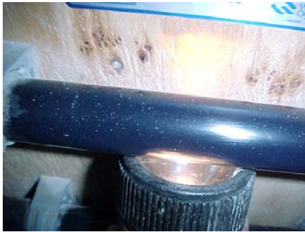
Black biofilm coating before application of mixed oxidants
