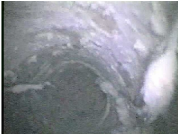
Feed water pipe with sodium hypochlorite
